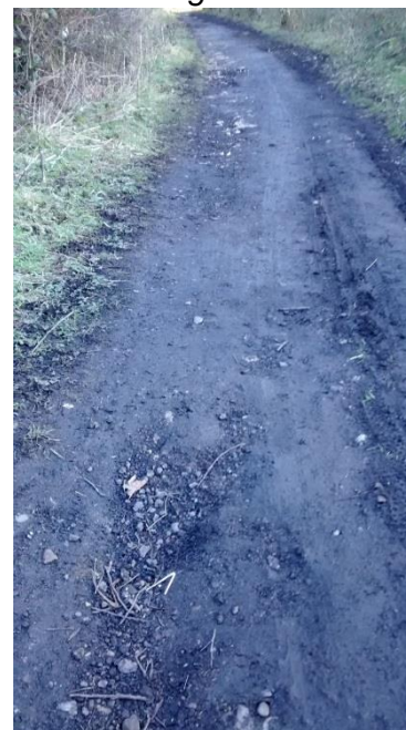
Water damage near Stainsacre
