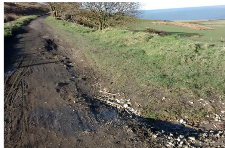
Water damage near Bay Ness
